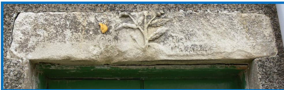
Figure 39 lintol at 14 New Street
