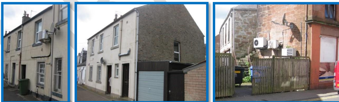
Figure 63 examples of unsympathetically located services detracting from the historic fabric
