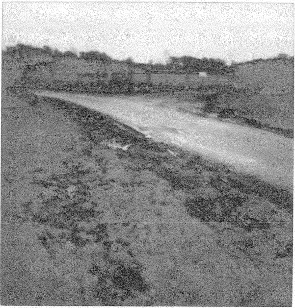
Dec 04 - Roadside kerbs still not replaced on New Mill Rd
