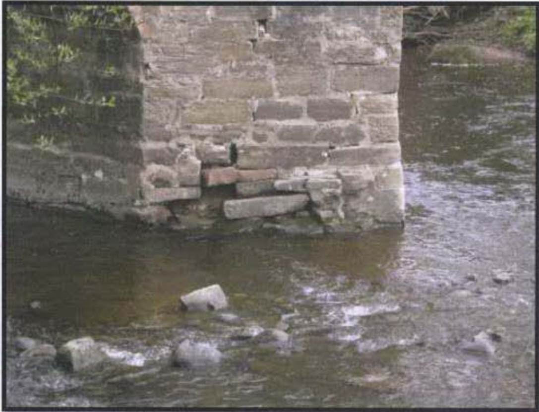
Photo 1. Missing Masonry / Damage at Upstream LHS of Cutwater.
