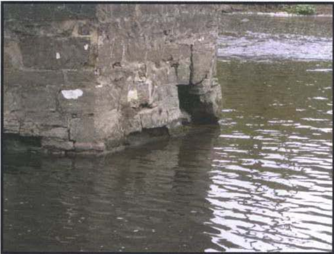
Photo 2. Missing Masonry / Damage at Downstream RHS of Cutwater.
