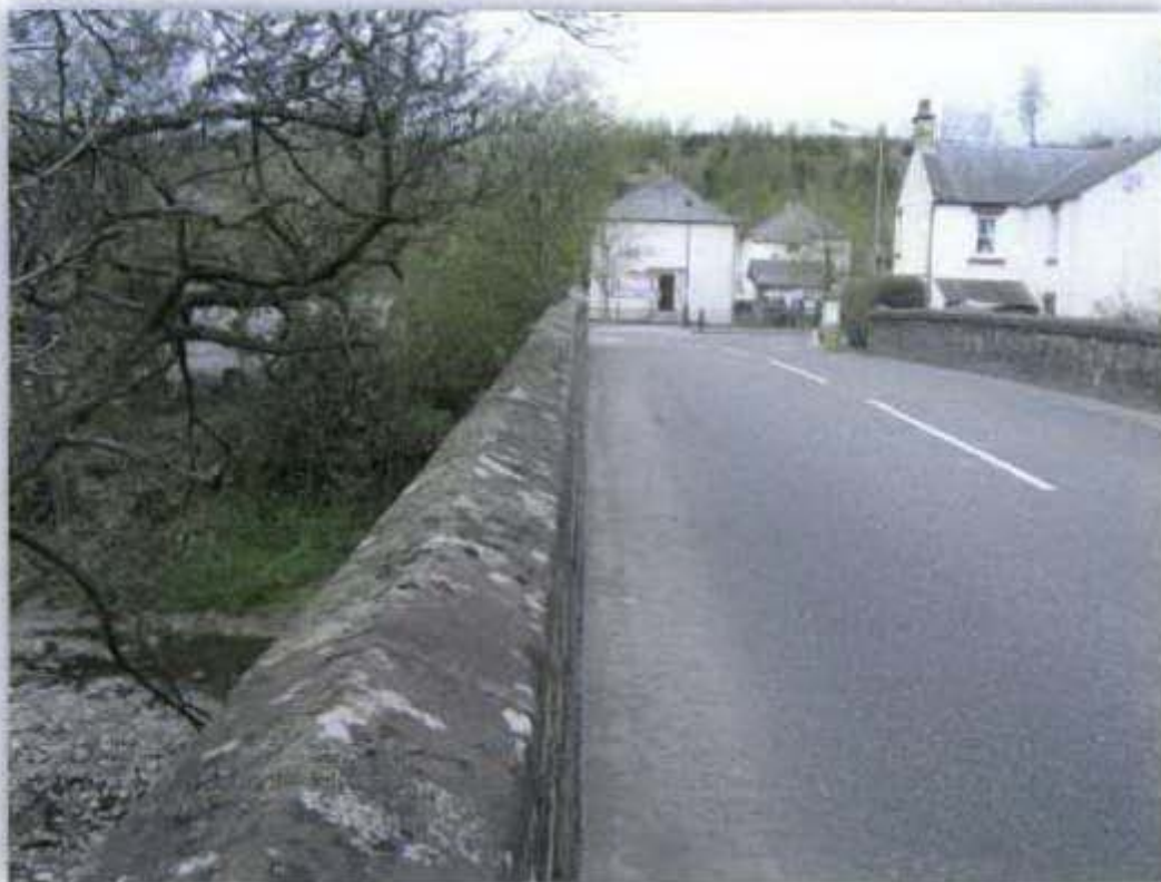
Photograph 2: Downstream Parapet leaning over towards river
