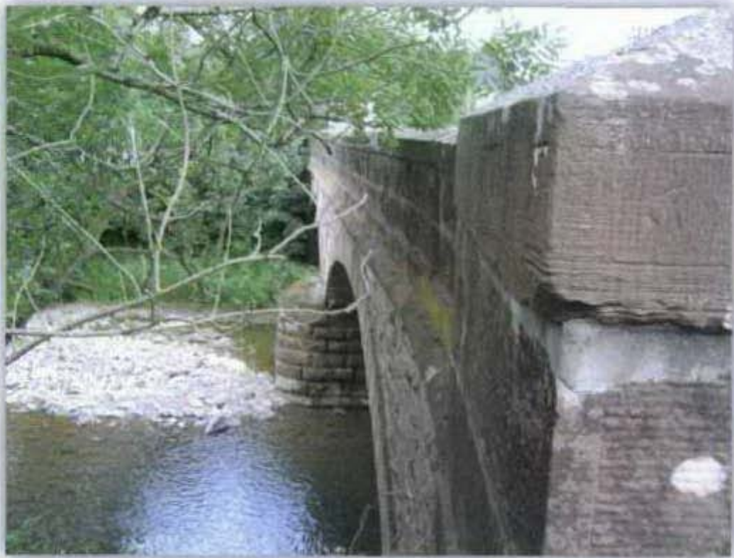
Photograph 1: Downstream Parapet leaning over towards river
