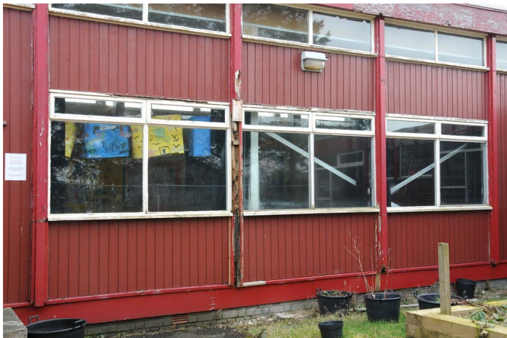
Photograph 2 : View into the Gym/Dining Hall with a view of structural timbers which have been exposed to view the extent of decay.
