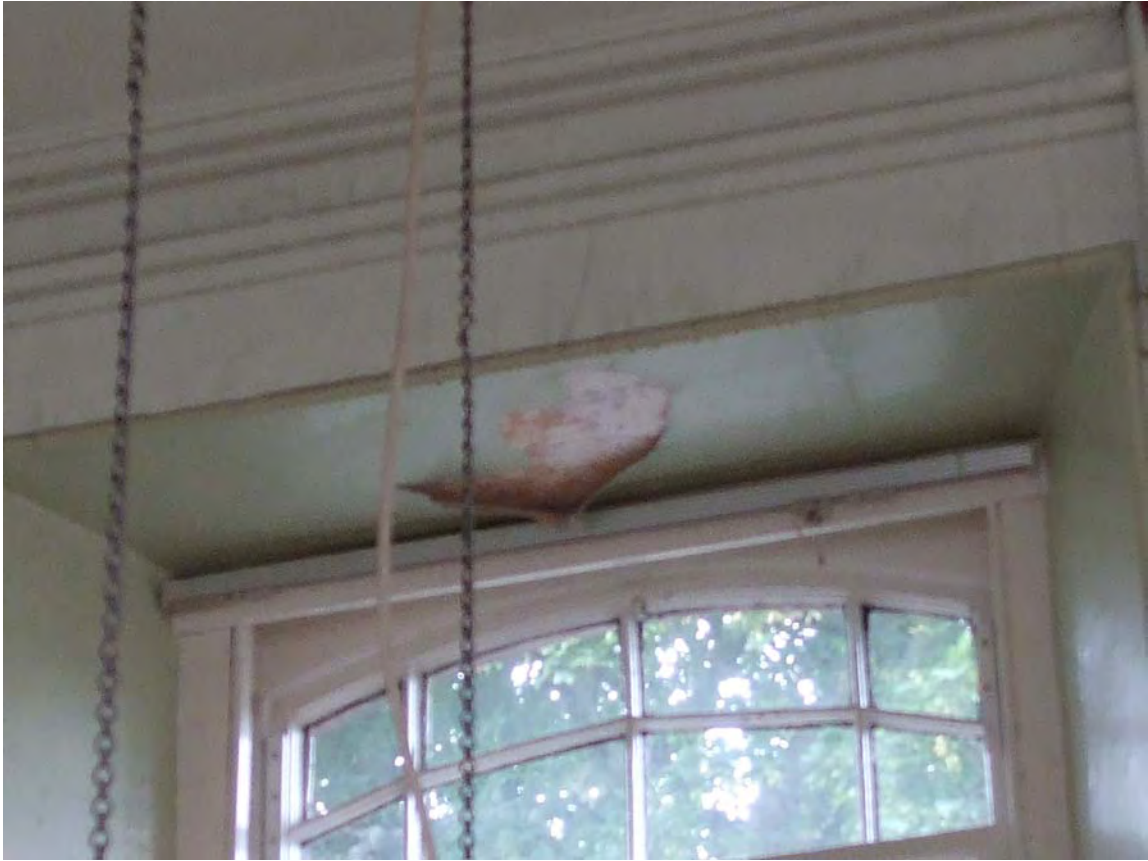
Photo 3: Deterioration of internal décor; high ceiling and dated windowline, Darvel Nursery School.
