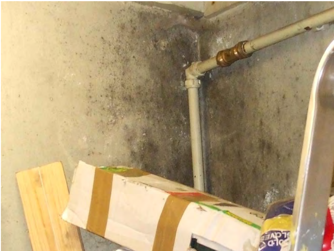
Photo 2: Ingress of dampness in cupboard, Darvel Nursery School.
