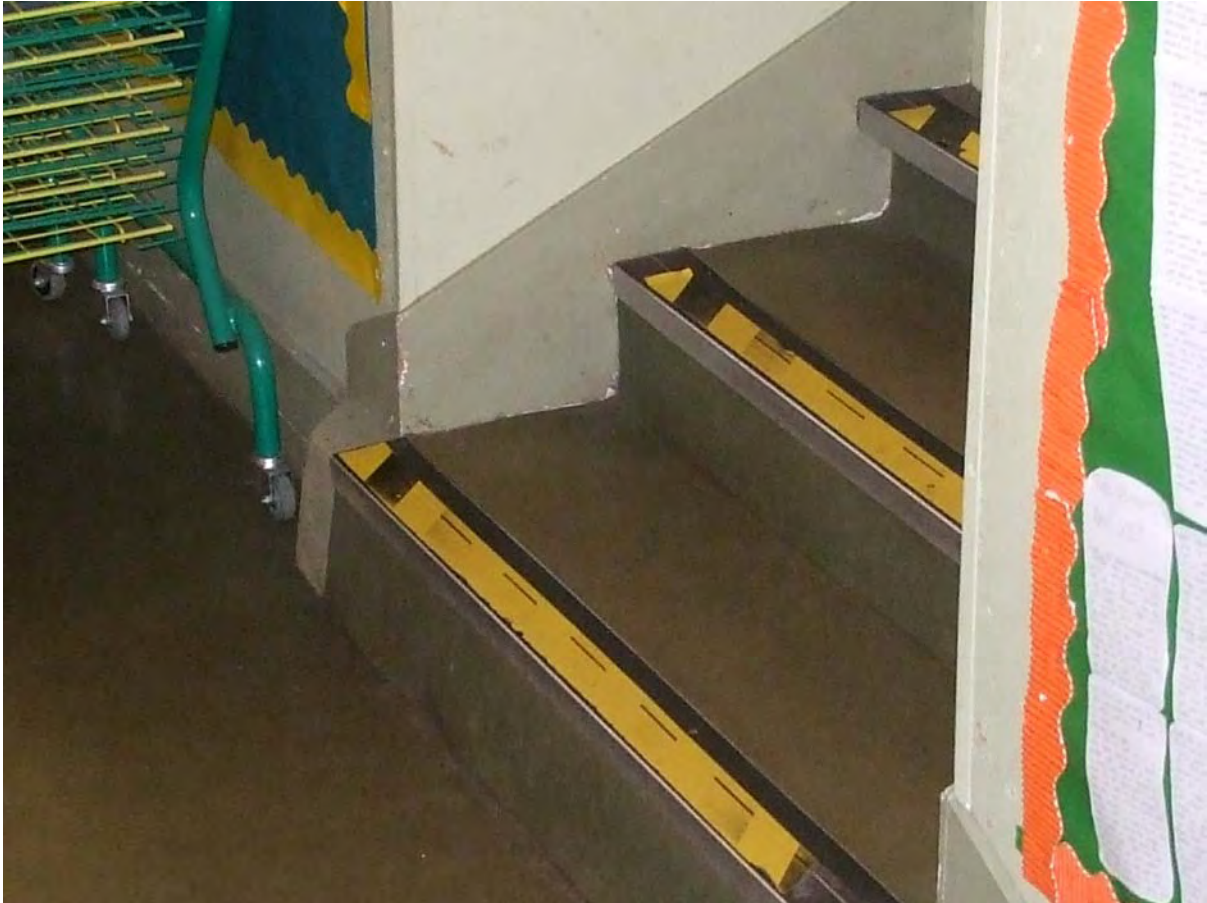
Photo 4: Restricted accessibility caused by internal stairs, Darvel Nursery School.
