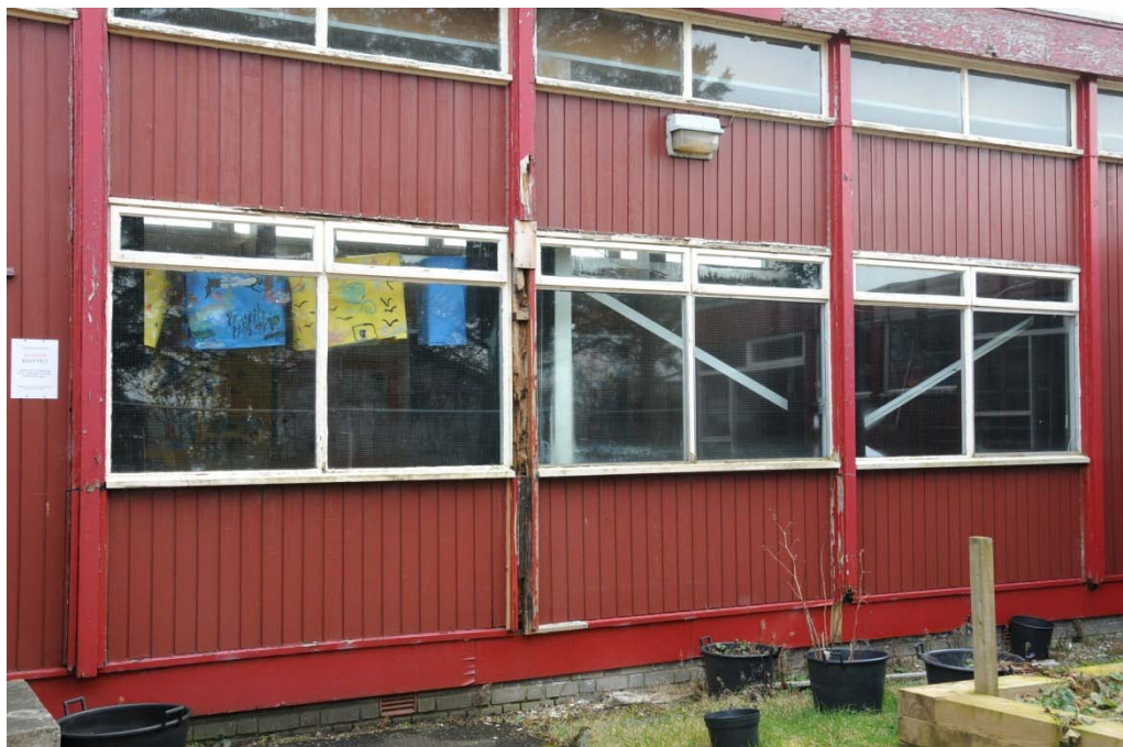
Photograph 2 : View into the Gym/Dining Hall with a view of structural timbers which have been exposed to view the extent of decay.
