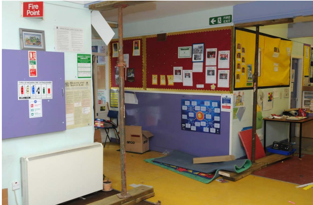
Photograph 3 : Corridor Area front at entrance. Internal roof supports can be seen in the foreground
